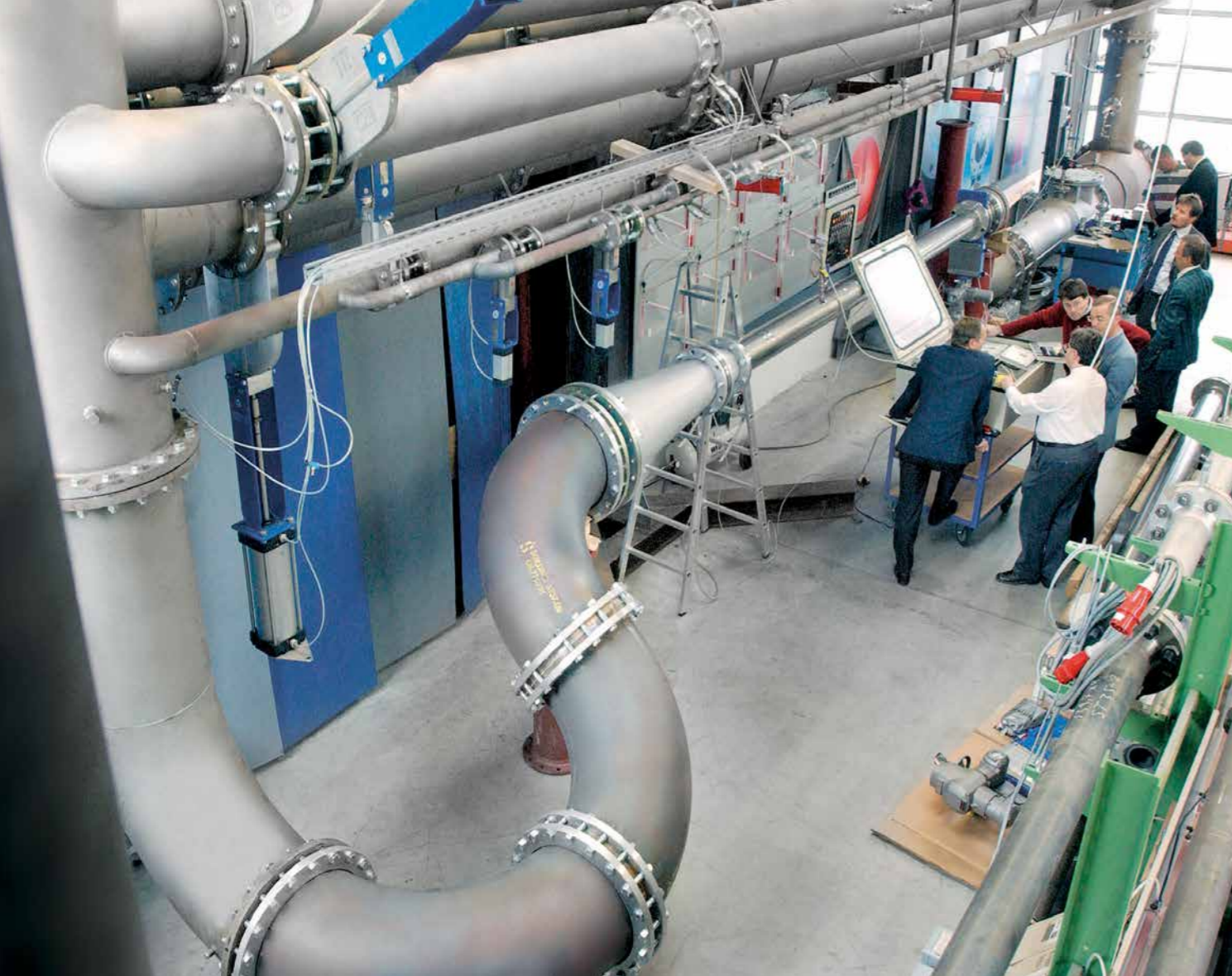
Factory approval testing (FAT) of the VACOMASS® air supply systems for the municipal sewage treatment plant of Vienna in our CAMASS® Calibration Lab. Due to the precise simulation of the field operating conditions and its piping layout during the calibration of the VACOMASS® systems, a field accuracy of 1.5% of the air flow reading could be guaranteed despite the difficult piping.
